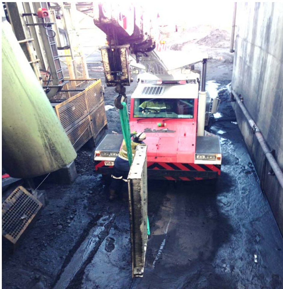
Figure 8 – The recovered second bottom deck plate
