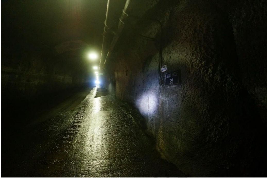
Figure 5: View to the portal up the drift from manhole 22 (Access to water and air services are next to the sign)
