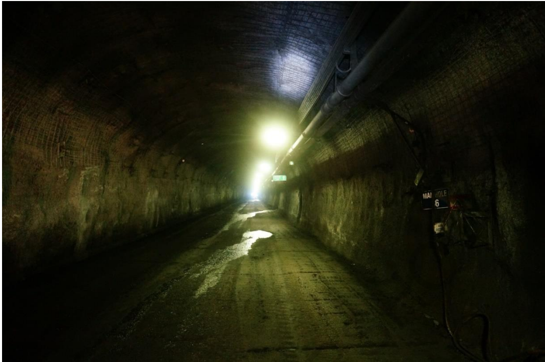
Figure 3: View up the drift towards the surface from near manhole 36. (Services pipes, including air and water, are in the top right quarter.)
