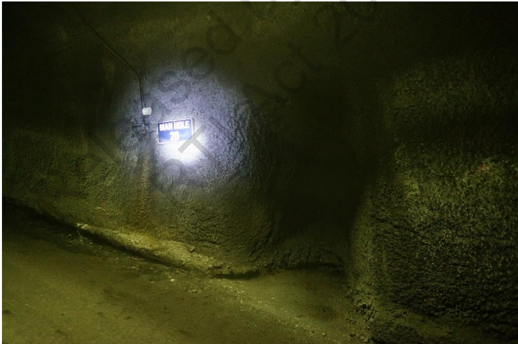
Figure 6: View of manhole 20 (Access to water and air services are next to the sign)
