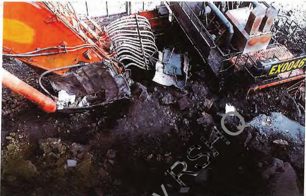
Figure 8. The incident scene post emergency rescue being completed
