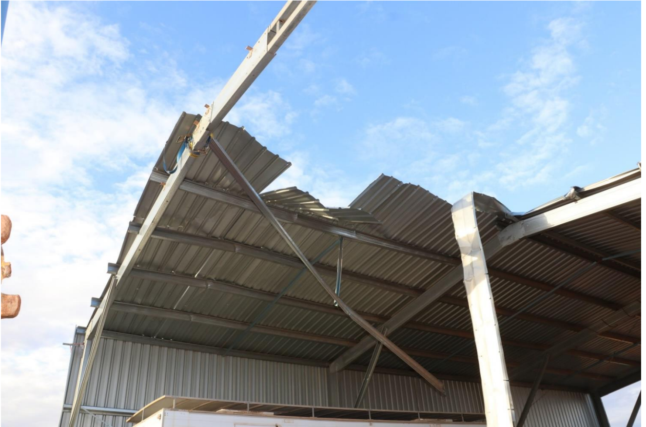
Photo 2: Section of roof structure where Mr Selig was working at time of accident
