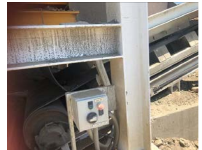
IMG_1225: CV0 Local Control Station (LCS)
