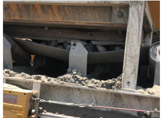
IMG_1276: Material falling off CV2 at transfer chute. Idler missing and skirting worn.
