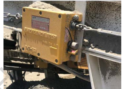
IMG_1299: Pull Wire Switch on CV2
