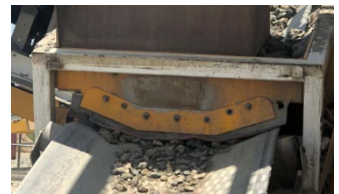
IMG_1309: CV2 - Lug for holding tail pulley guard broken on LHS
