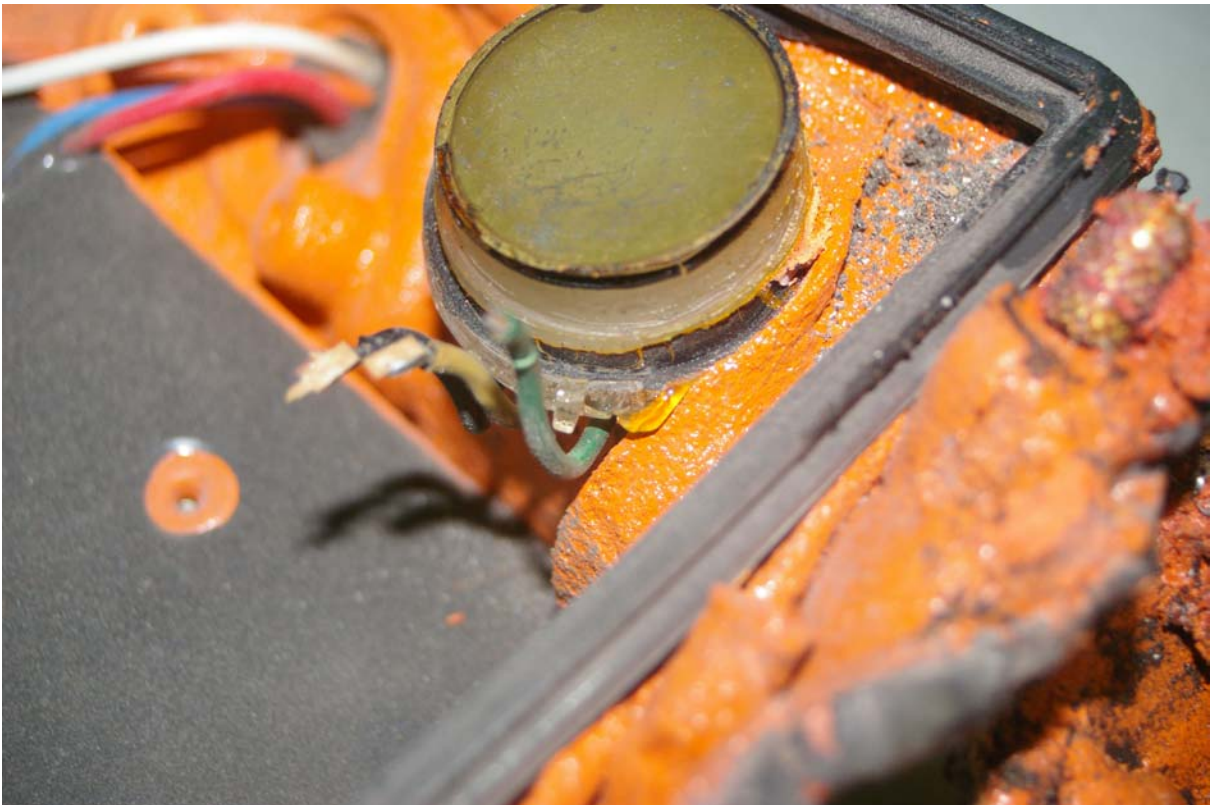
Photo 8 – internal wires detached during separation of boards
