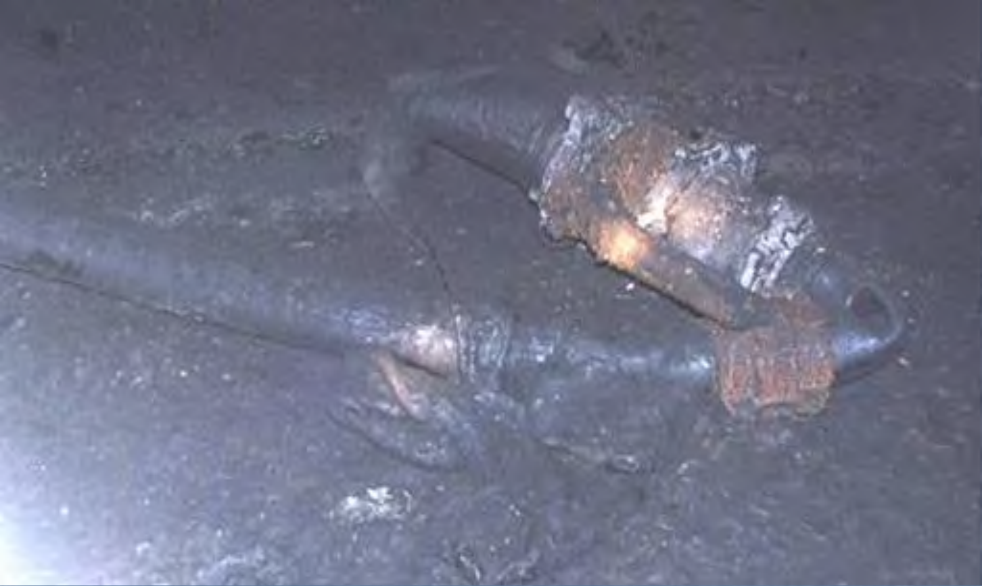
SL4 Travel Road 3-4 C/T : Poly Pipe with steel valve
